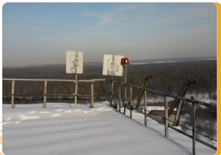
SkyMAN R5000 base stations on the roof of one of the ARMS
